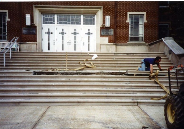
Photos circa 1992— Sister Mary Virginia Wamfler, CSA moving out of her wing to make room for construction to begin; Demolition of the front steps in preparing the transition of Mt. Augustine to a health care facility.
